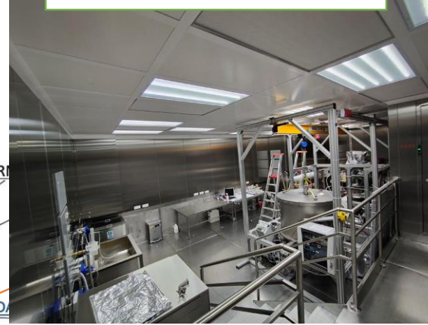
CR1 Radon free clean room
