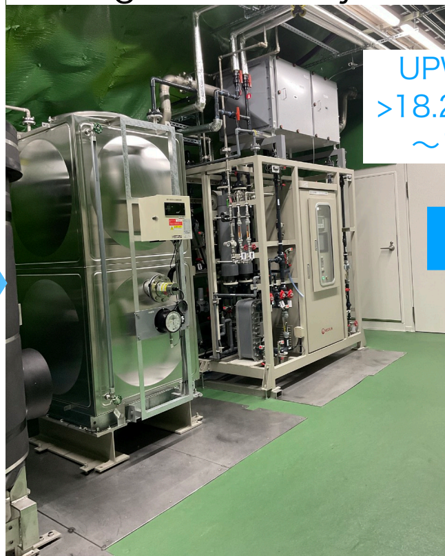
UPW generation system
