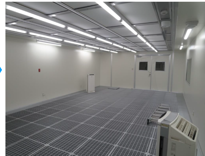
Super clean room
