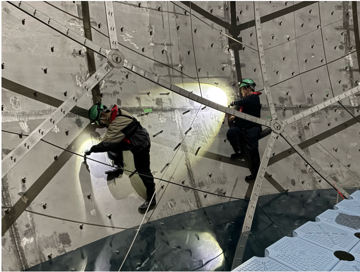
Broken bolt removal from boss
