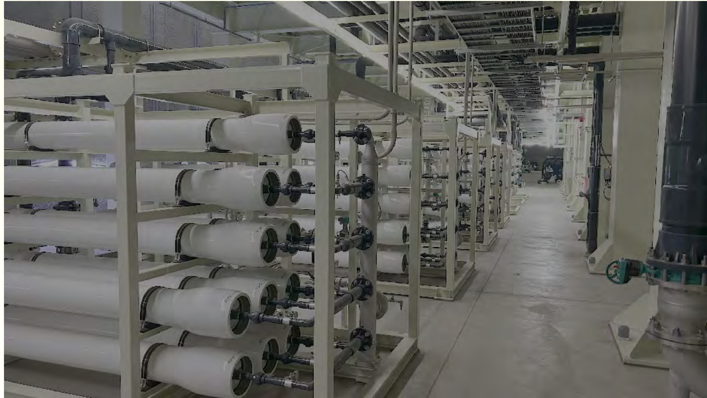
Water system already installed and waiting for operation
